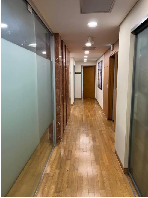
Corridor from Main Door leading to Consul General’s Office (with obvious discoloration of wood parquet due to previous year’s Embassy roof water leak incident)
