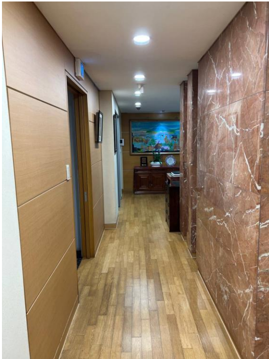
Corridor from the Main Door (with obvious discoloration of wood parquet due to previous year's Embassy roof water leak incident)
